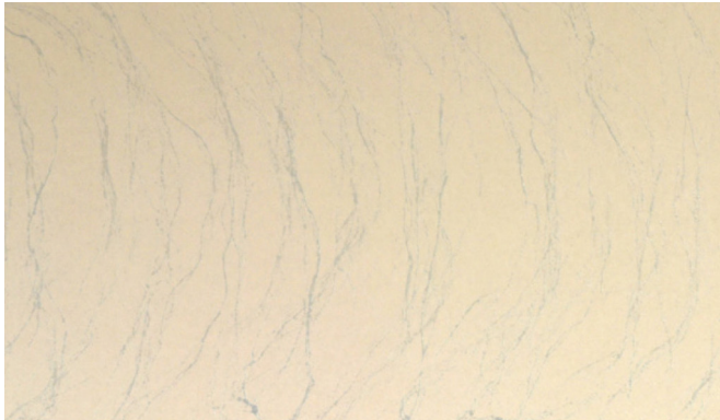
COVERAGE TOO LIGHT
